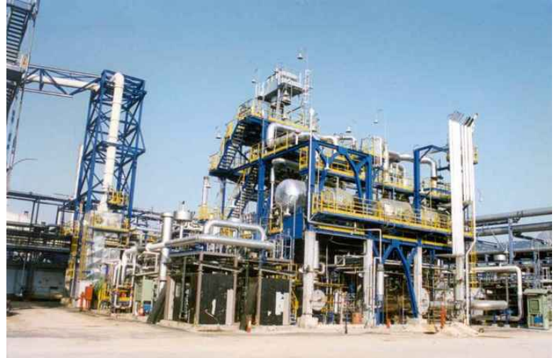
Hellenic Aspropyrgos Refinery – Gasoil HDT & Sulfur Recovery Units
